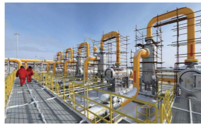
China-Russia East-Route Natural Gas Pipeline
